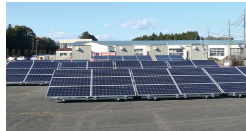
Test combining PV panels and solar inverters
